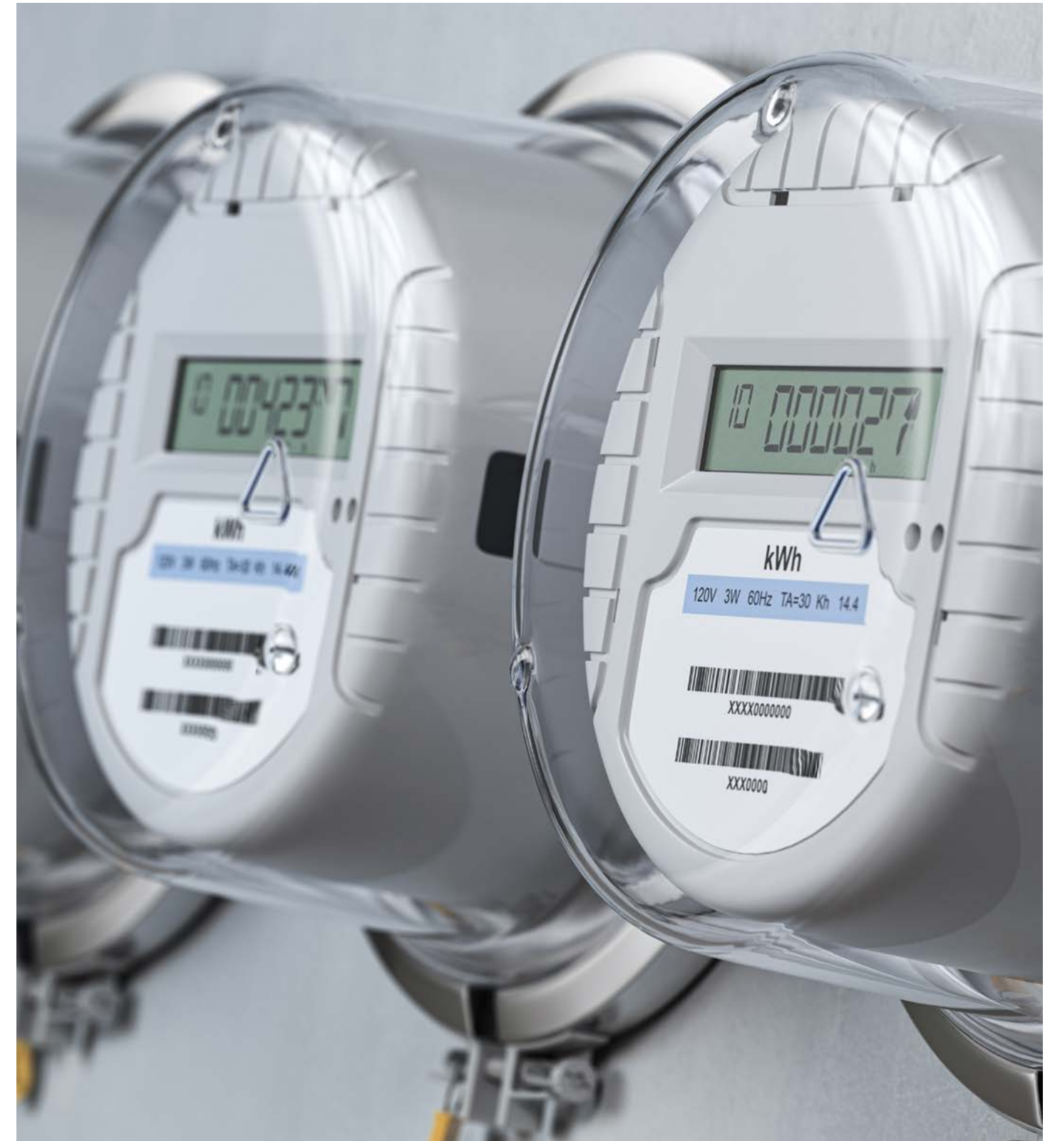
Building energy meters.
